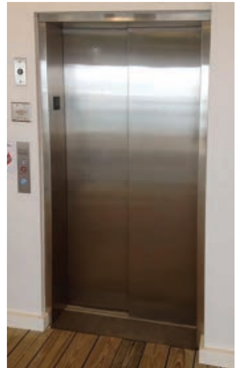
Brushed Stainless Steel landing door
